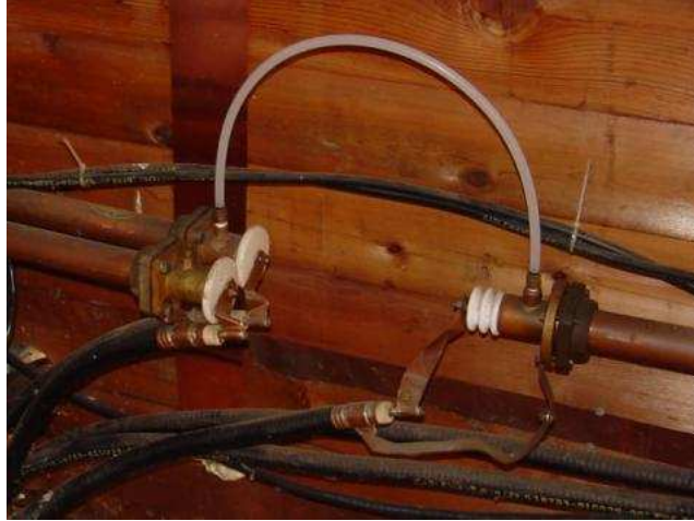
Figure 14.52: Flexible coaxial cables connected to rigid lines.
